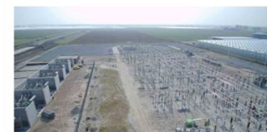
MS-MS station (3-23kV)
